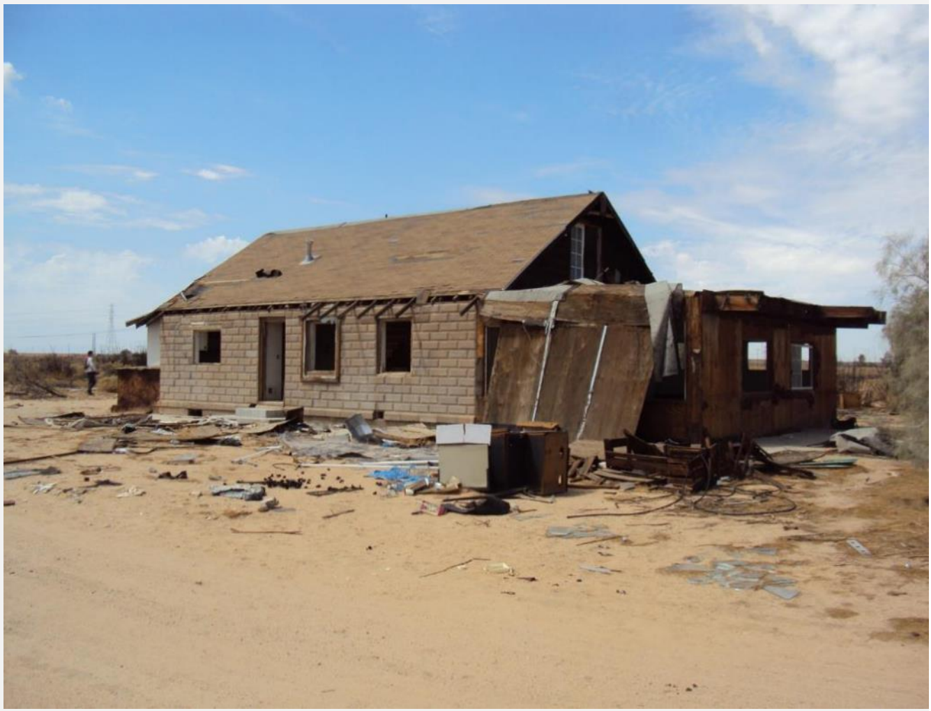
Exhibit 5-1. View of residence at ranch complex in northwestern corner of Project site; view to southwest.
