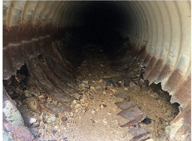
Photo 1. Mile 4.7 deteriorated culvert (February 18, 2025).
