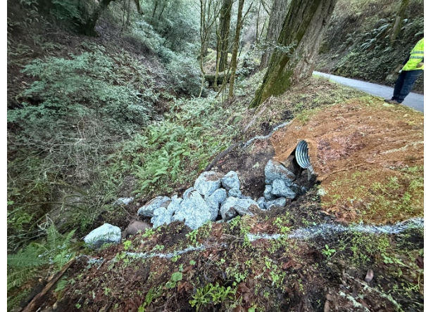
Photo 1. Slip-out facing east (2/20/2025).
