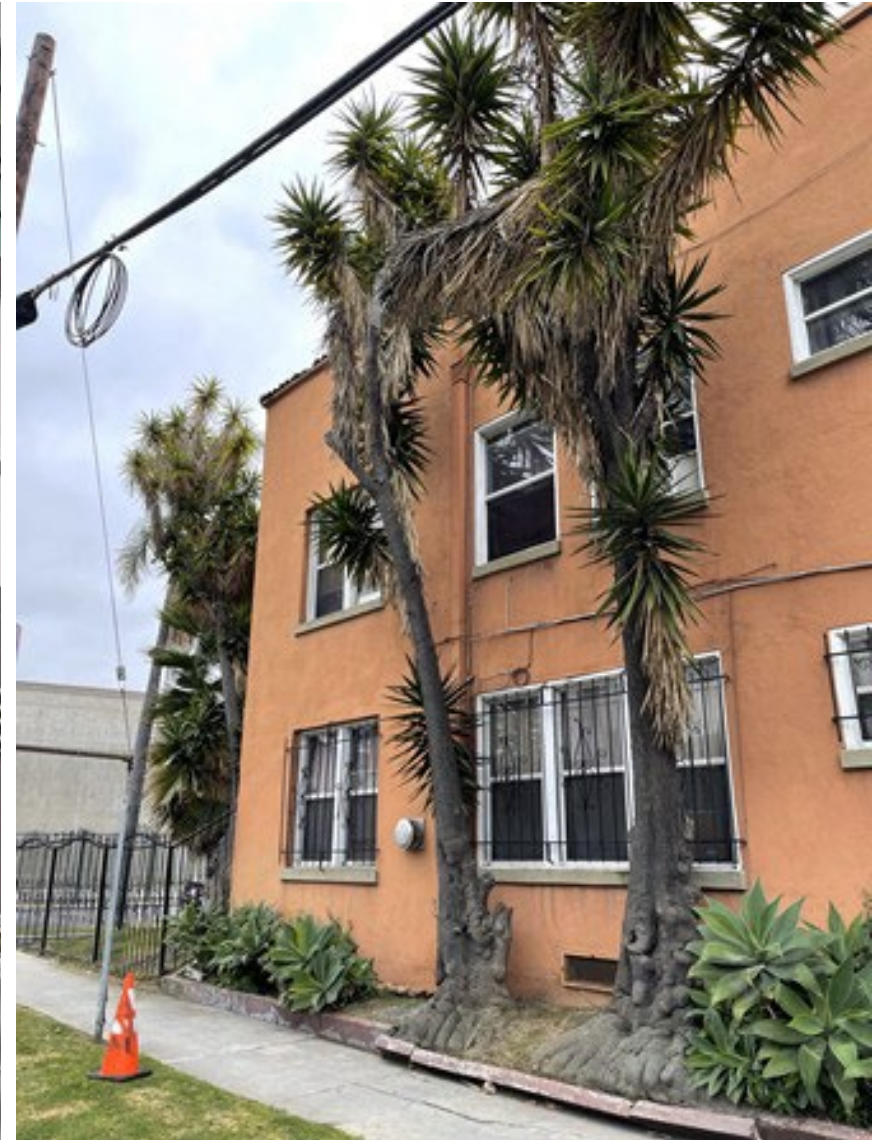
#4 & 5 Yuccas with #6 around the corner. Note root damage.
