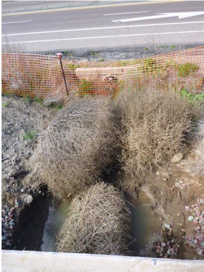
Photo 13. Ponding immediately after culvert
