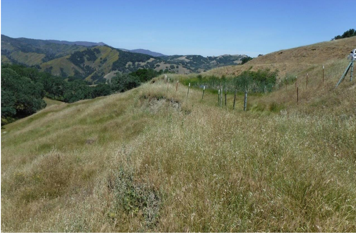
Photograph 5. The eroding berm below the fence at RC-07, facing west.
