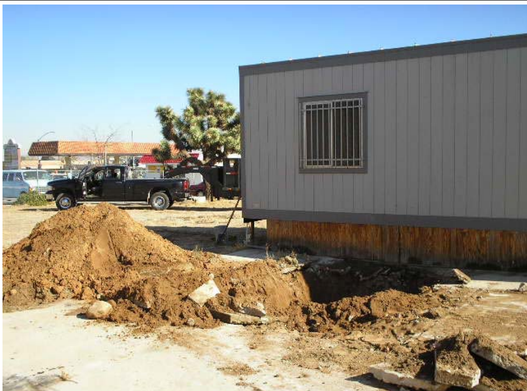
Photograph Number 8: Hydraulic lift removal excavation behind portable building in SW corner.
