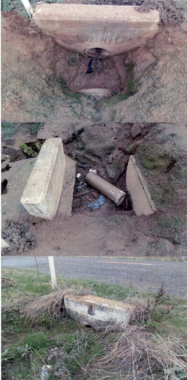
Headwall for Culvert 1. The headwall and pipe are constructed of concrete, the pipe may be transite but determination is difficult. The form impressions indicate this is a poured concrete structure and not precast. The pipe at the bottom of the photo is metal and travels under the roadway. The pipe diameters range from 1 foot to 1.5 feet.
