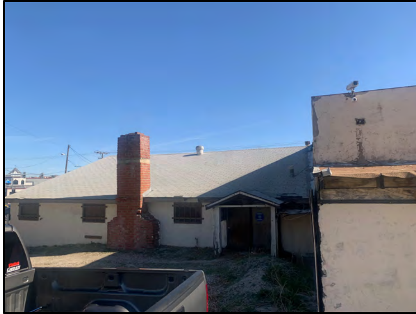
Figure 9: Overview of the remnant 1920s home, showing how it is embedded in the current structure (facing northeast).
