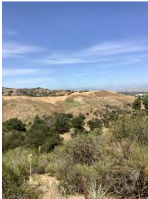
Figure 4. Southern view of vegetation in Project area, and active construction work occurring just outside of the western Project boundary.
