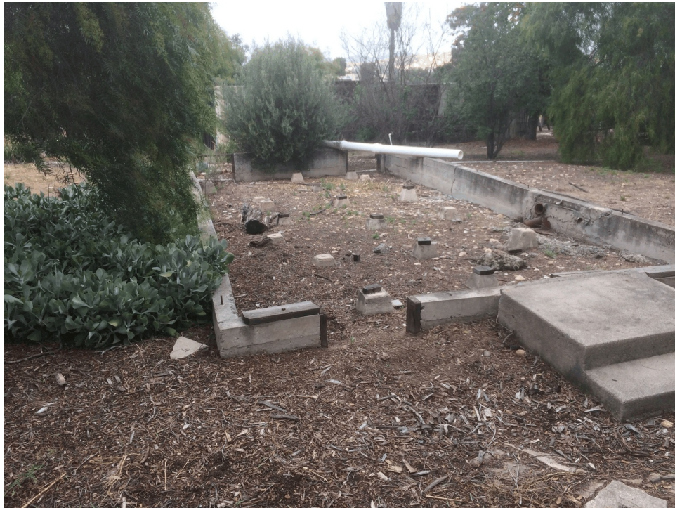
Photograph 10: View of a small building foundation near the south-central portion of the Property, looking northward
