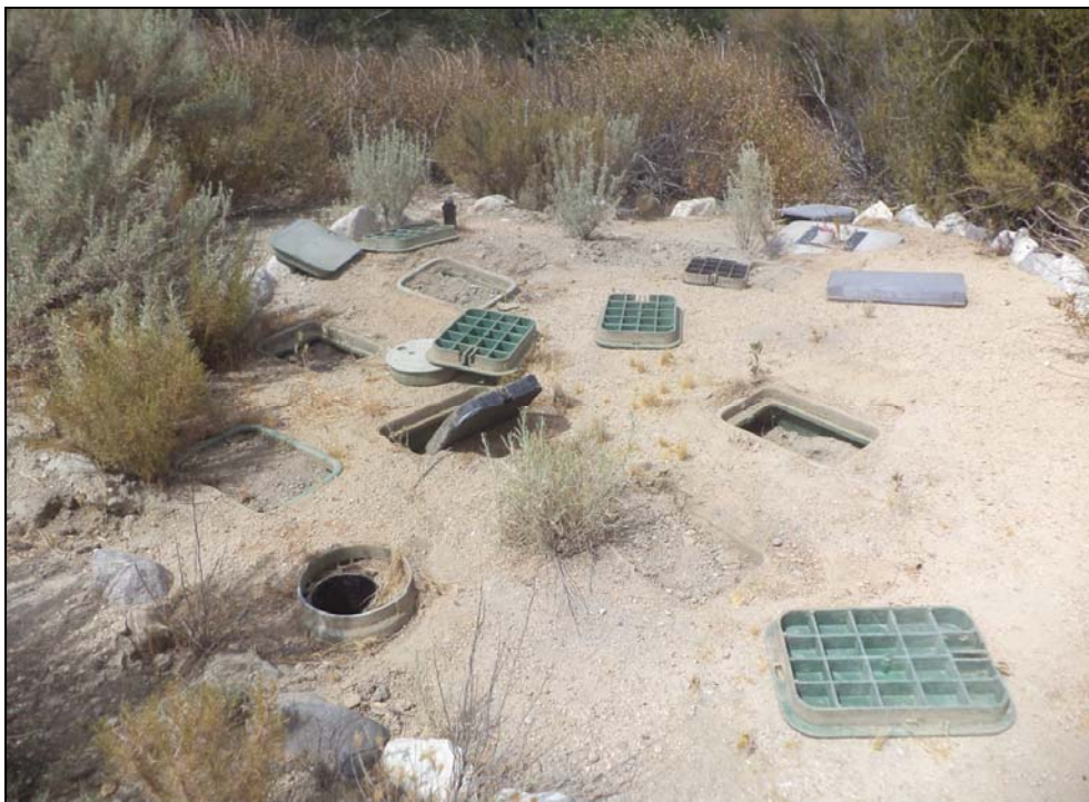
Photo 12: Typical view of electrical utility boxes throughout the site which have been dismantled with wires exposed.
