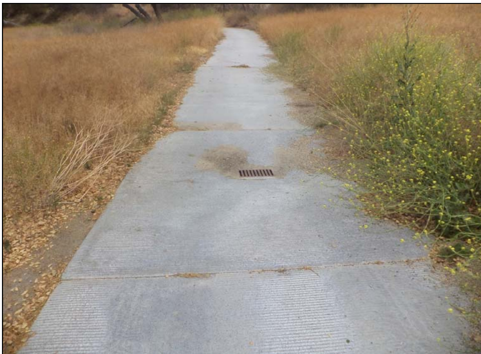
Photo 16: View of a storm water drain within the golf cart path on the western portion of the subject property.
