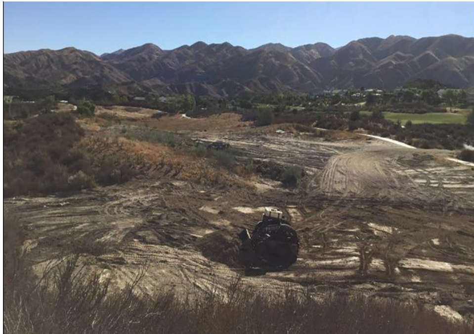
Figure 5. Overview of Easternmost Section of Proposed Project Site with Visible Grading Activities. View Facing East.
