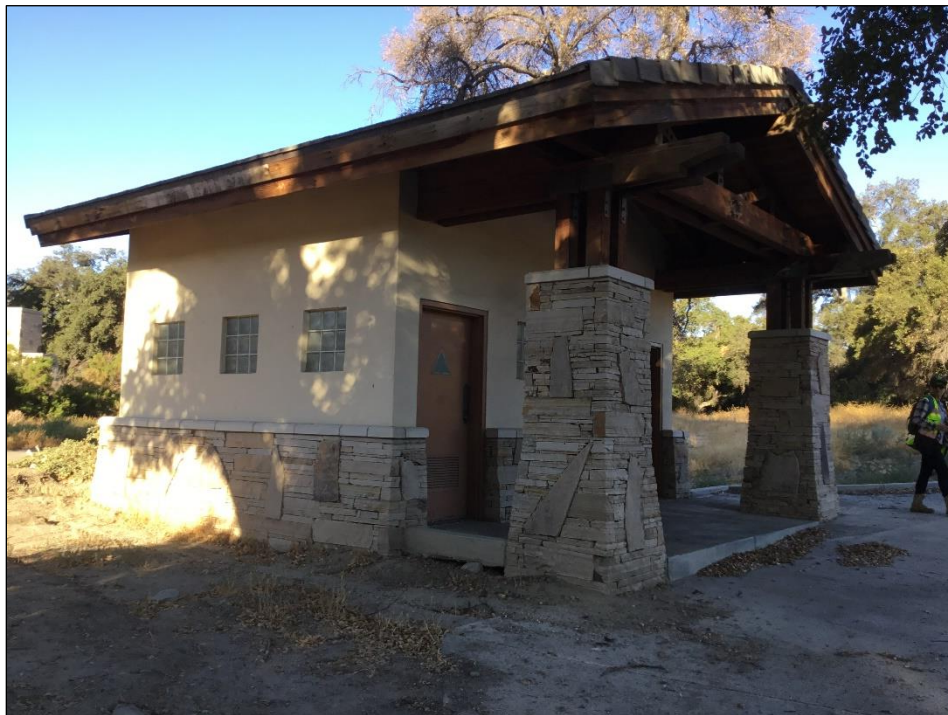
Figure 9. Abandoned Restroom Located at Southwest Corner of Proposed Project Site. View Facing Southwest.
