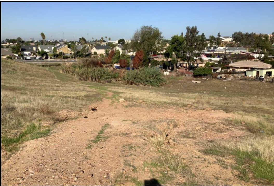
PHOTOGRAPH 2 Eroded Area, Looking Northwest
