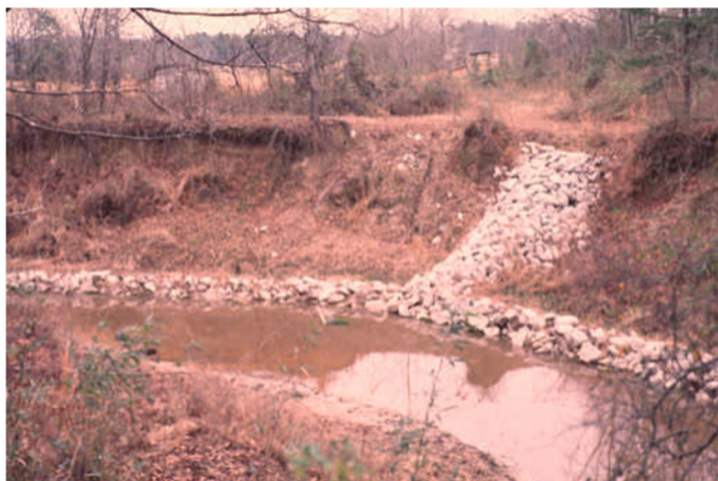
Figure 3. Photo depicting a tieback similar to those designed for SR Erosion Contract 4 (USACE 1997).
