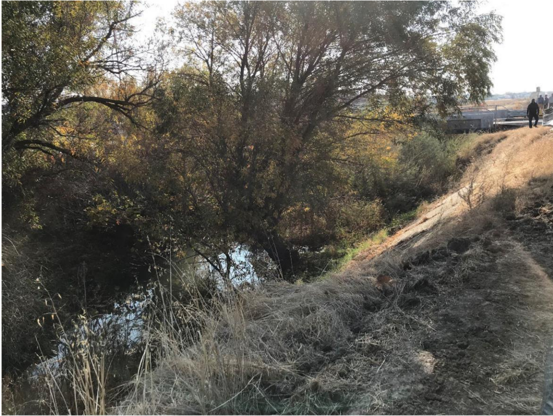
Photo 11: Looking Upstream at Vinci Ave. Bridge Downstream Face, Tree in Channel Noted
