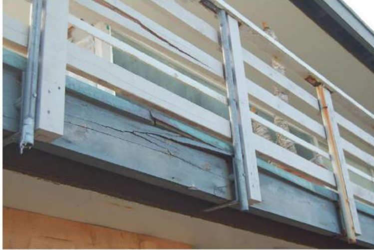
Deterioration and splitting at deck edge.
