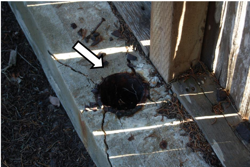
Photo 29 Location of removed fence support post.
