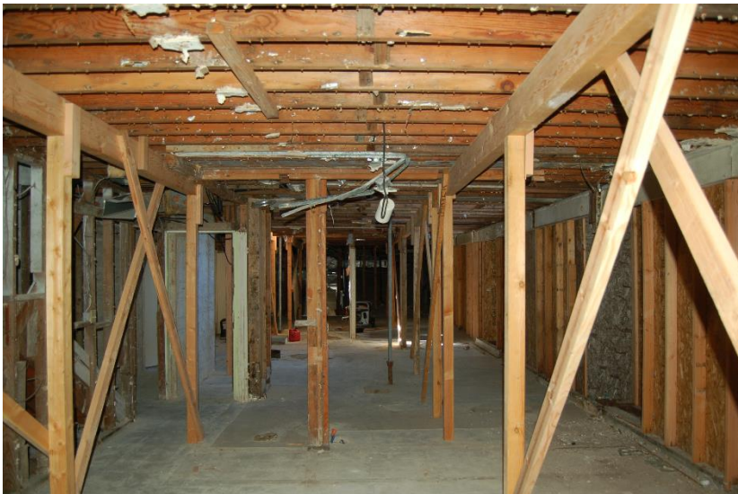
Photo 24 Lower level has been gutted of all finishes and the upper level floor is supported on two rows of wood shores.
