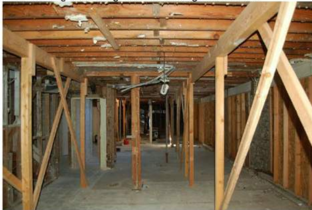
Lower level has been gutted of all finishes and the upper level floor is supported on two rows of wood (temporary shoring).
