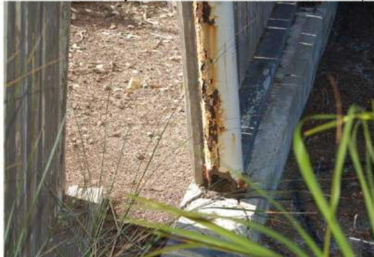
Hole at base of cantilever pipe fence support and spalling of concrete curb.
