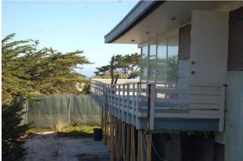
Temporary shoring installed. Note sagging deck and handrail along upper level west face.
