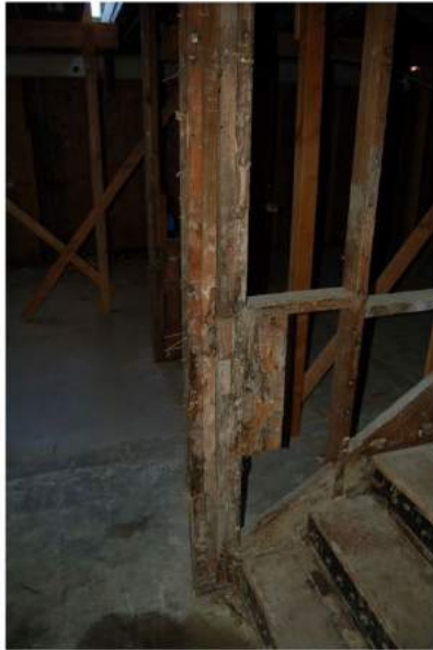
Water staining and damage to wood framing at lower stair.
