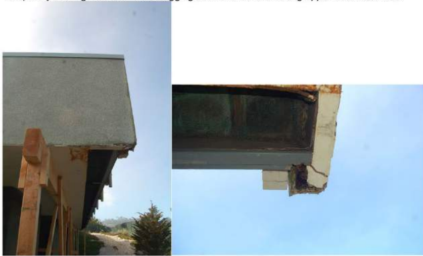
Framing deterioration is evident at the northwest corner of the deck.
