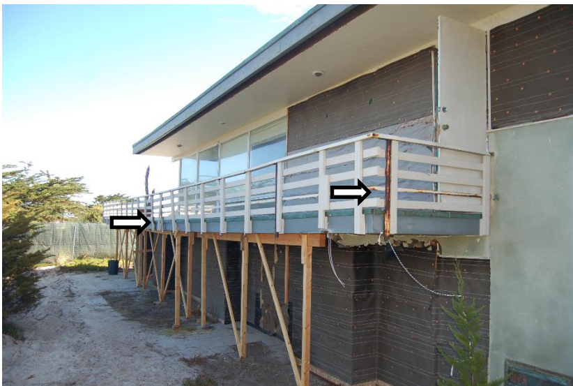
Photo 10 Rusted steel hand rail posts and wood replacement posts that are failing in some locations.
