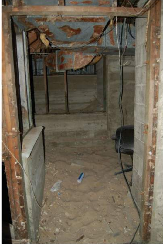
Rusted ventilation system ducts. Note that floor slab is not present in mechanical areas.
