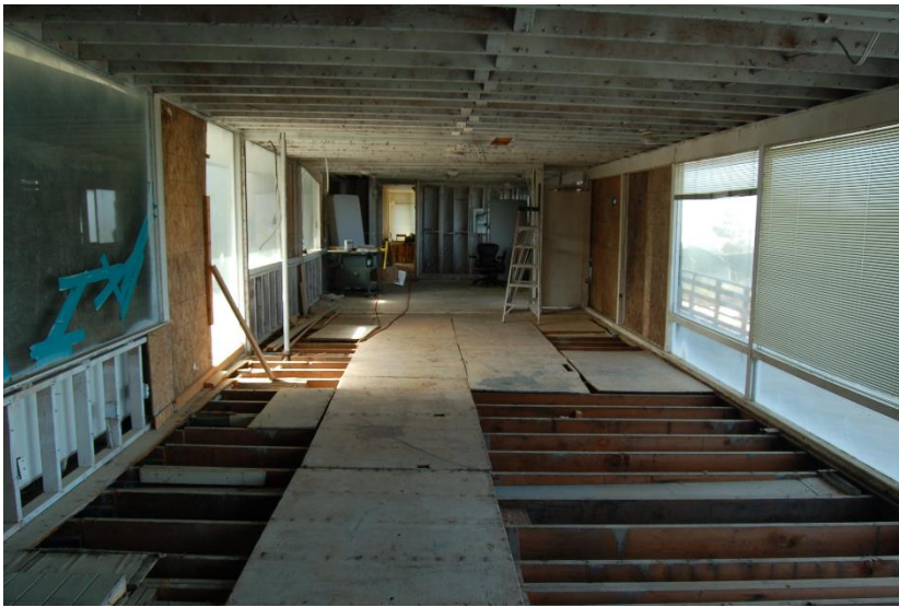
Photo 19 Upper level floor framing, saw cut at both ends and supported by shoring below.
