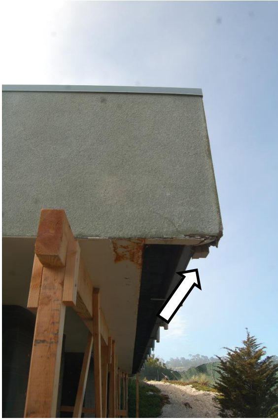
Photo 11 Framing deterioration is evident at the northwest corner of the deck.
