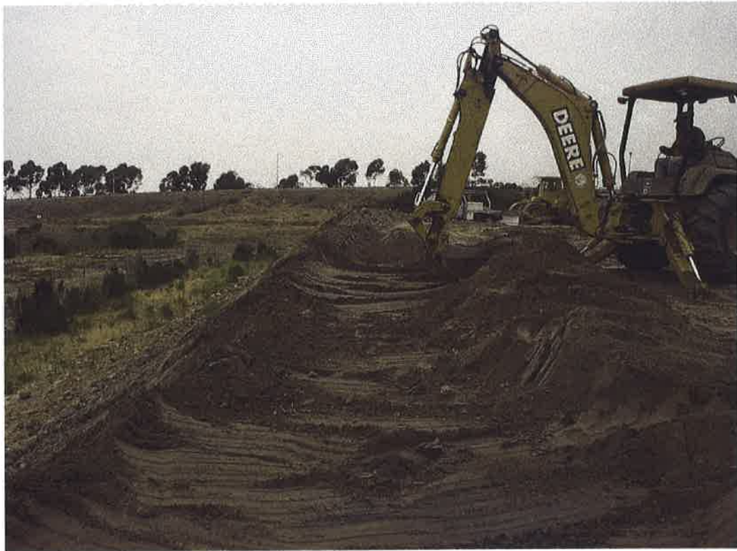
Backhoe removing contaminated material from slope face on south side of stockpile.
