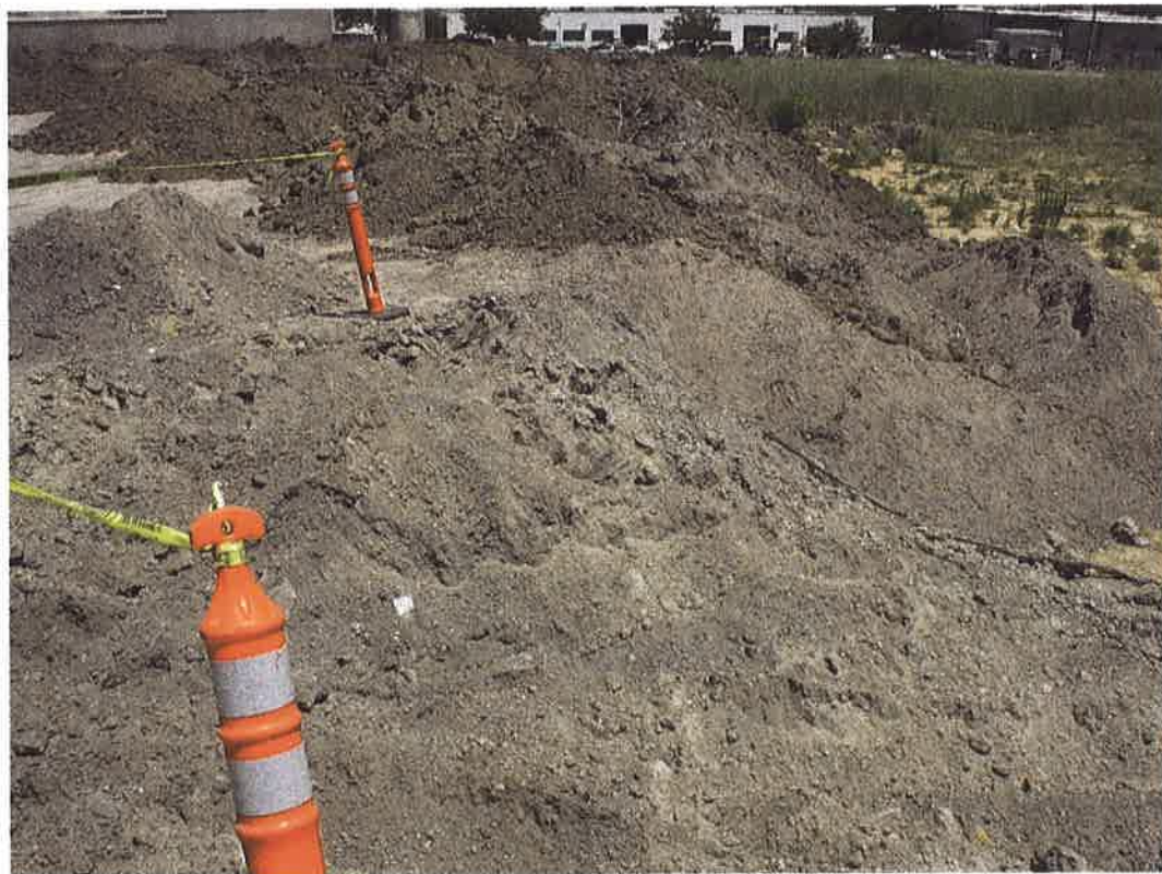
Additional excavation on south side of stockpile prior to re-sample of S-22
