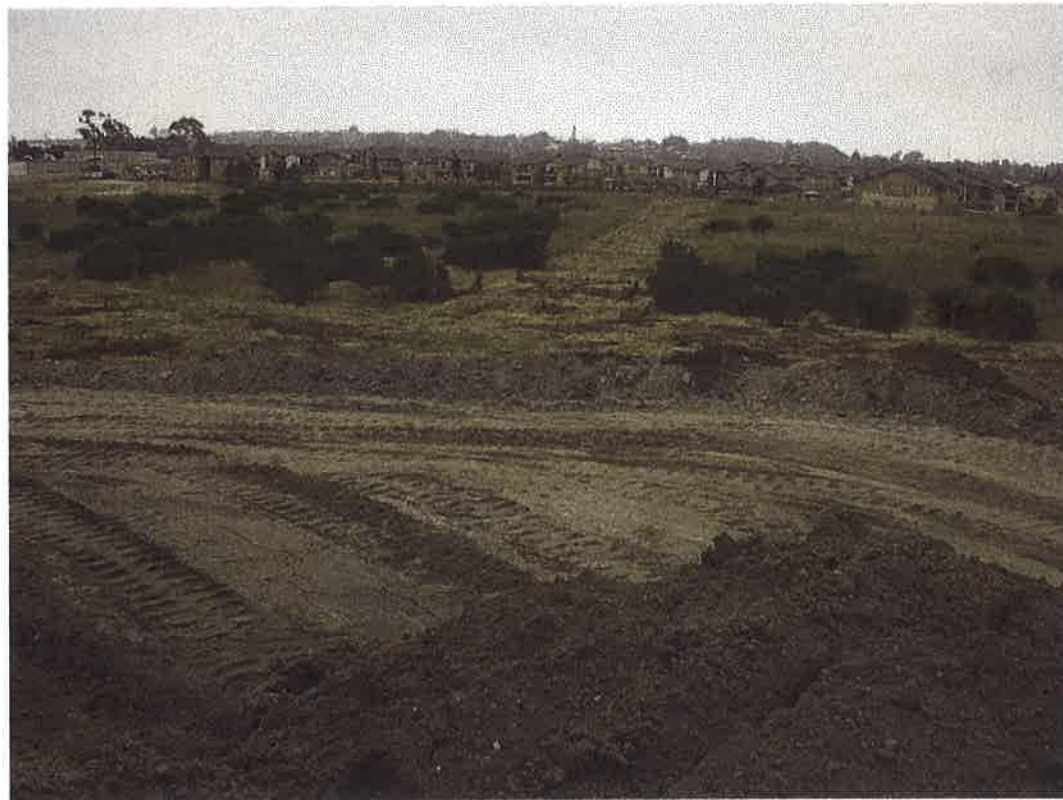
Looking south at berm along south edge of stockpile, prior to scraping.
