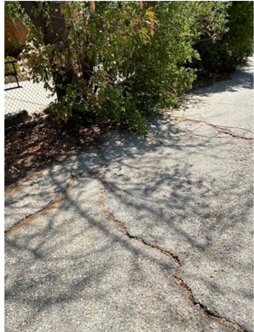
Note the damage caused by the ash roots.
