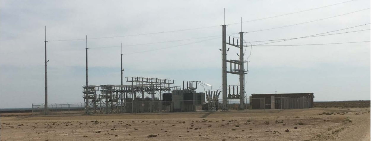
Figure A4. Typical Substation
