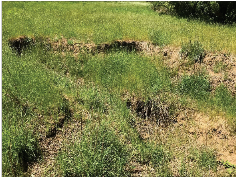
Photo 2: Example of an existing erosional gully (headcut) that would not be repaired due to Draft EIR mitigations
