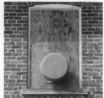
c. The exhaust fan has tamper-proof housing.
