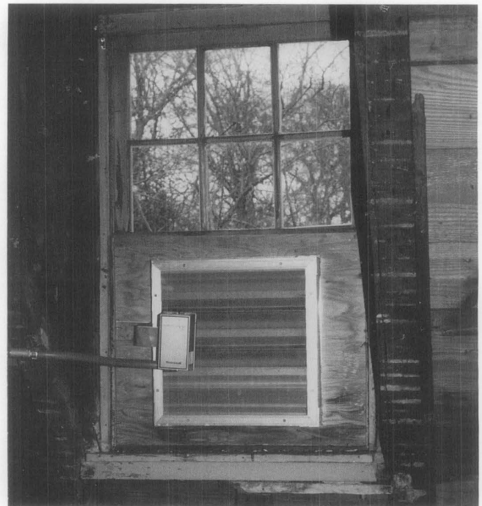
Figure 21. This electric thermostat/humidistat mounted in the attic vent controls a modified ducted air/fan system. The unit uses temporary exposed sheet metal ducts to pull air through the building and exhaust it out of the basement. For over ten years this fan system in combination with 18" x 18" preformed louvers in selective windows has kept the interior dry and with good air exchanges.
