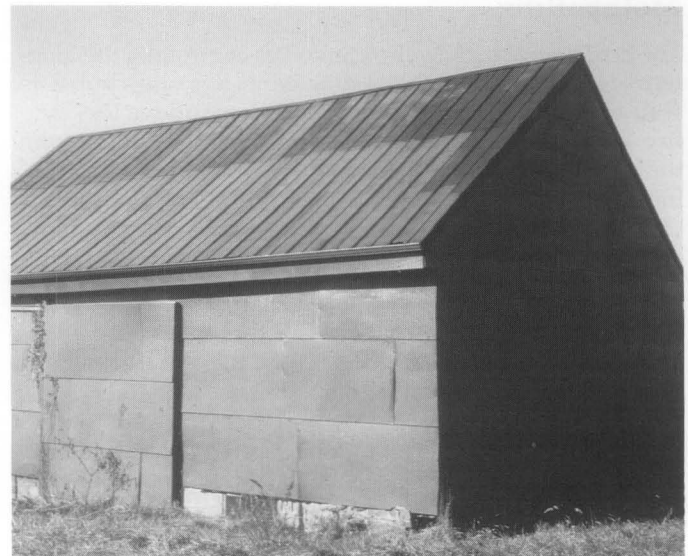
Figure 9. Severely deteriorated wooden siding on a farm building has been covered over with painted plywood panels as a temporary measure to eliminate moisture penetration to the interior. Foundation vents and loose floor boards allow air to circulate inside.
