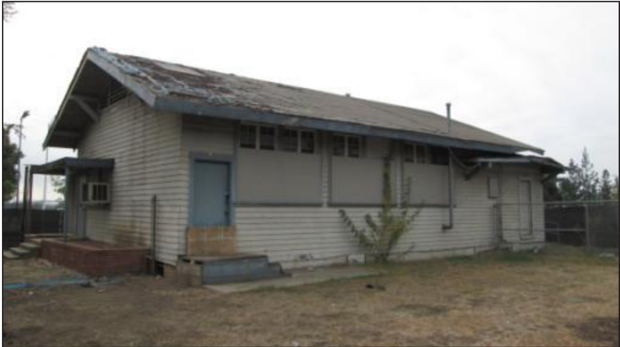
View of the Old Schoolhouse looking southwest. The entrance to the building is on the left (eastern side of the building). Note the physical condition of the building.
