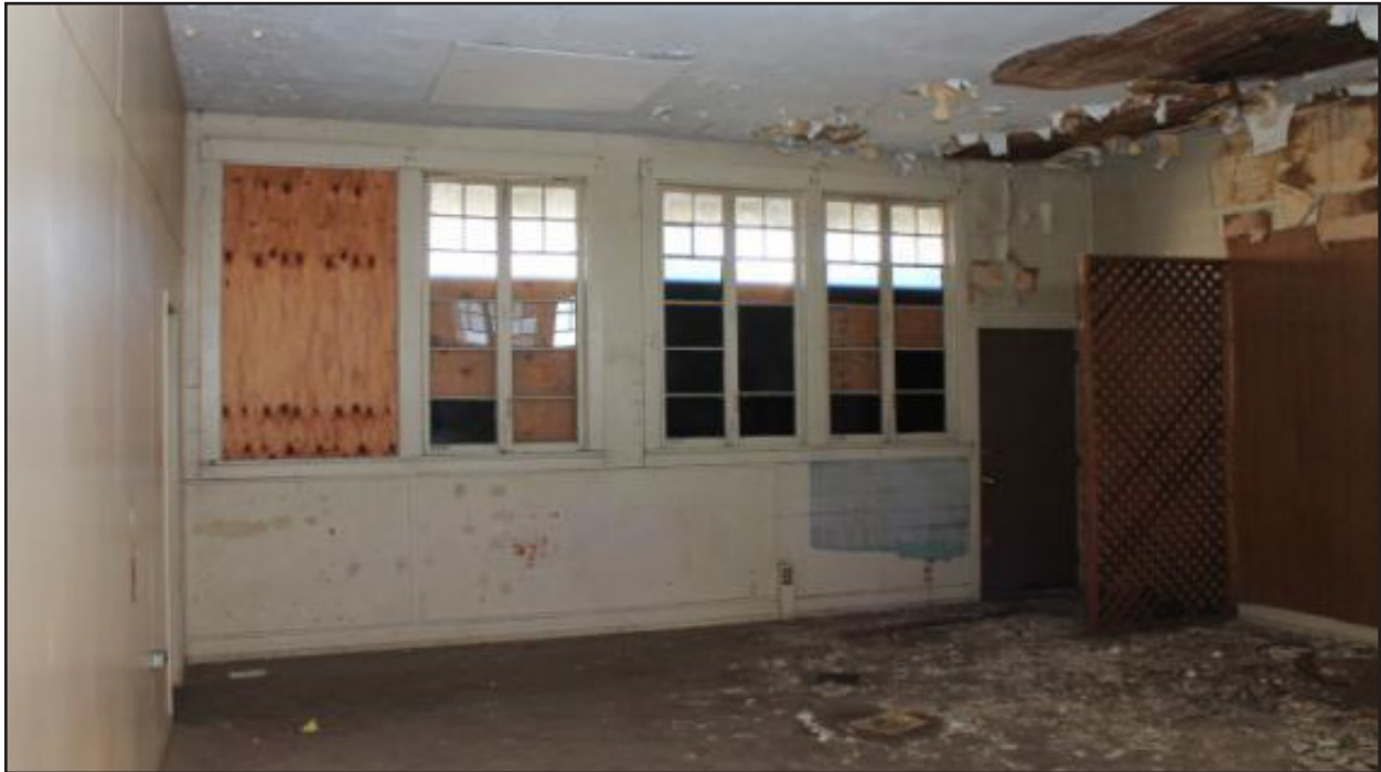
View of the north wall of the main classroom room. Notice the condition of the ceiling, walls, floor, and window fixtures.
