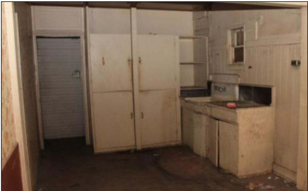
View of the kitchen and pantry area in the northwest corner of the building. Notice condition of the kitchen amenities and surfaces.
