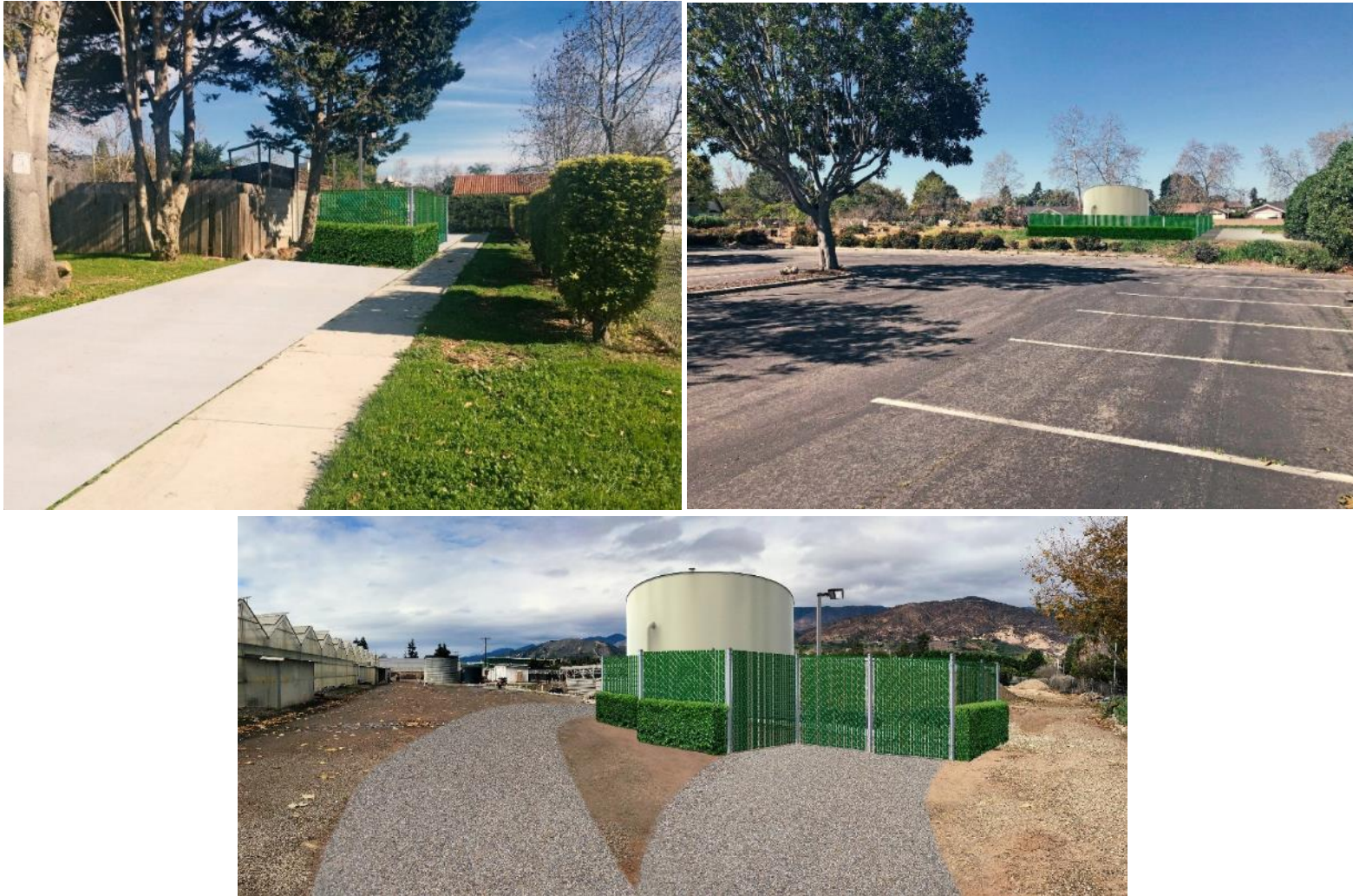
Top Left: Injection well at Well Site #2. Top Right: Injection well and tank at Well Site #4. Bottom: Injection well and tank at Well Site #6.
