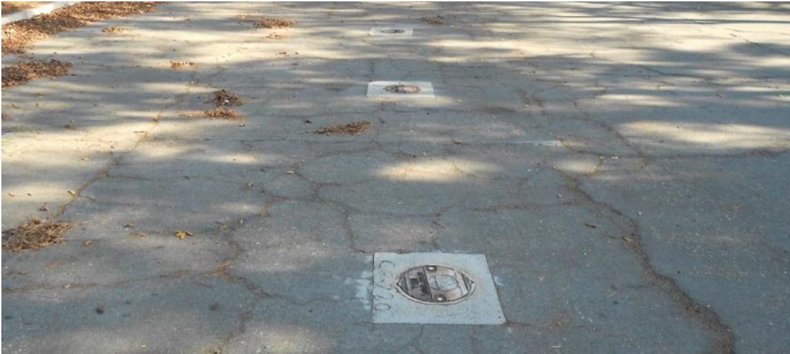
Figure 2-8. Example of Monitoring Wells
