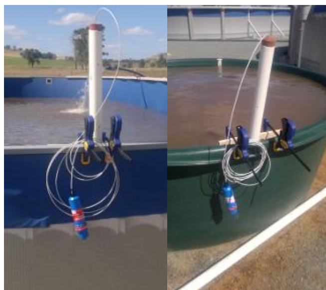
Figure 18: Odyssey’s capacitance water level sensor probe and the PVC shroud installed in the evaporation ponds and water troughs. (Photograph: A. Leung)
