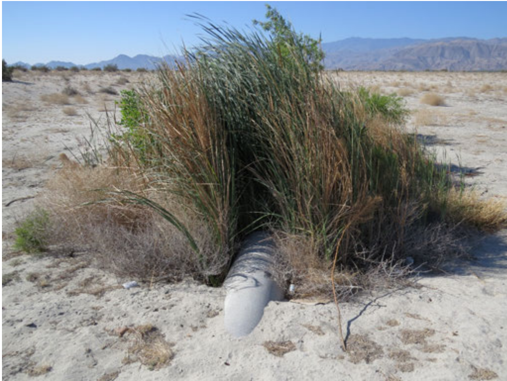
Photograph 11: Culvert that receives water from surrounding development on the northern boundary of the site that has created a stand of emergent vegetation.
