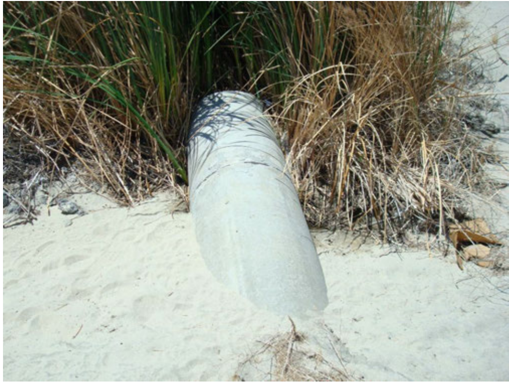
Outlet of 24-inch reinforced concrete storm drain pipe in Retention Basin "A" Photo 1
