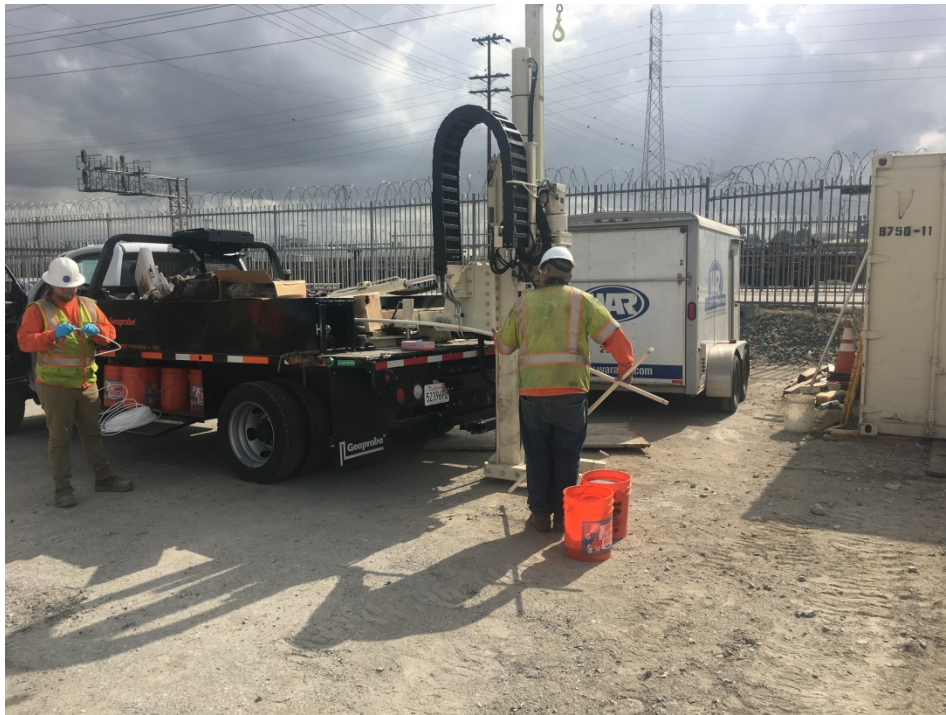
a. Direct Push Drill Rig with crew working on installation of Vapor Probe at 2A-3
