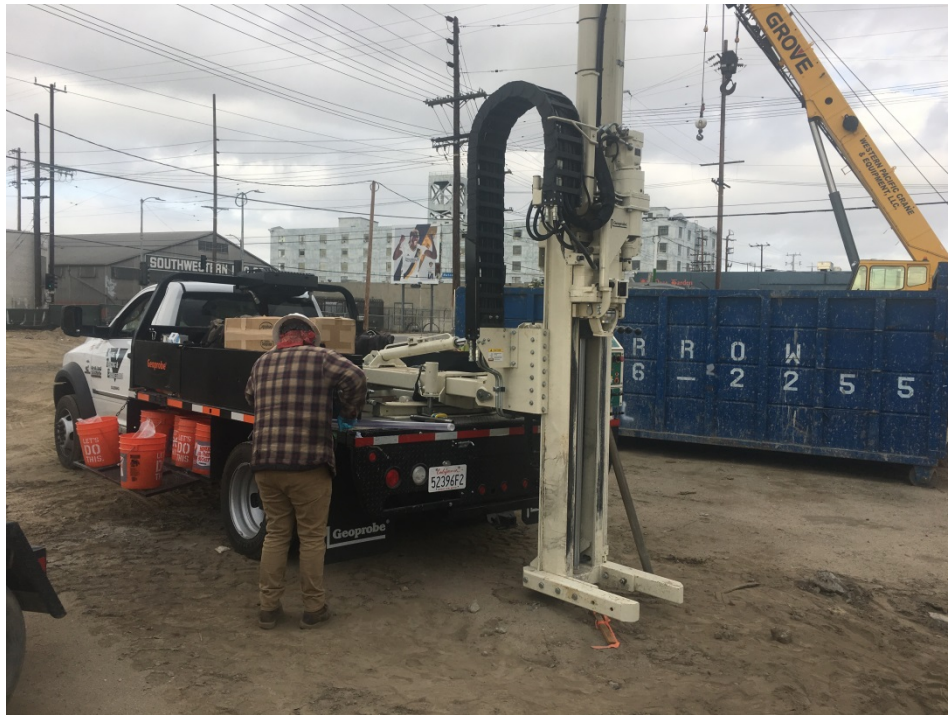
a. Direct Push Drill Rig with crew working on installation on sample liner
