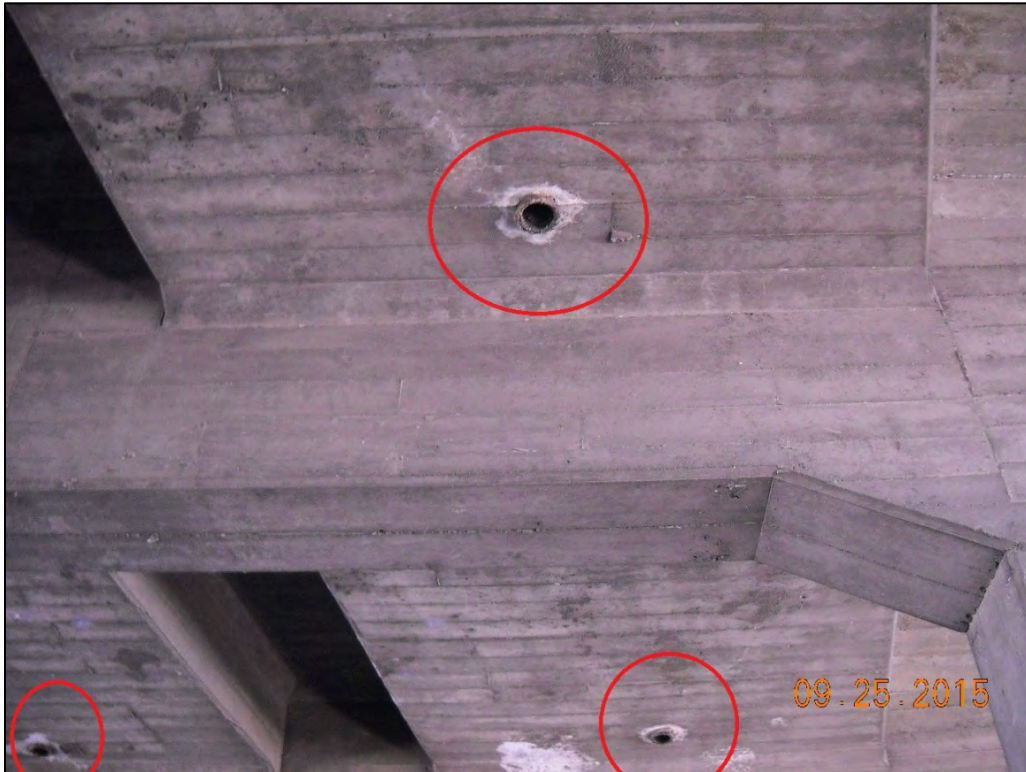
Photo 7: Drainage holes on the underside of the Seventh Street Viaduct upper bridge deck; view facing east
