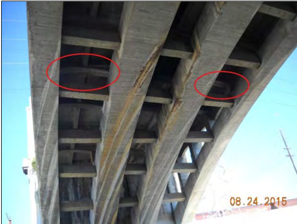
Photo 3: Underside of Fourth Street Viaduct showing eastern expansion joint; view facing east
