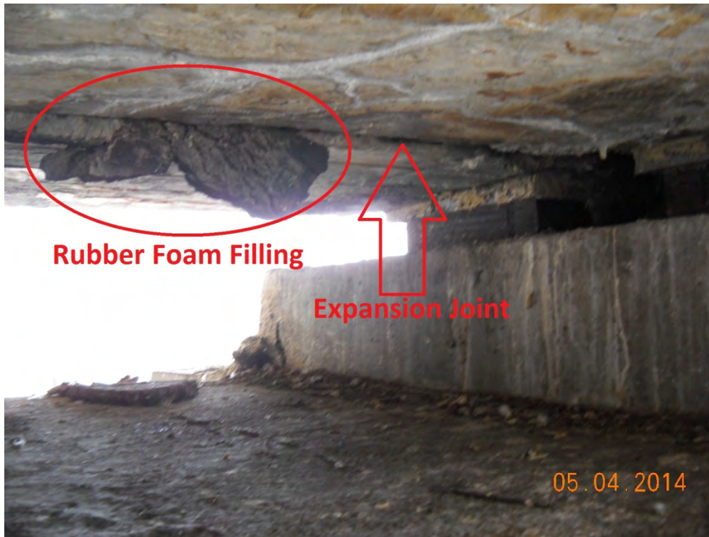
Photo 7: Falling rubber foam filling providing suitable bat roosting habitat within expansion joint; view facing west
