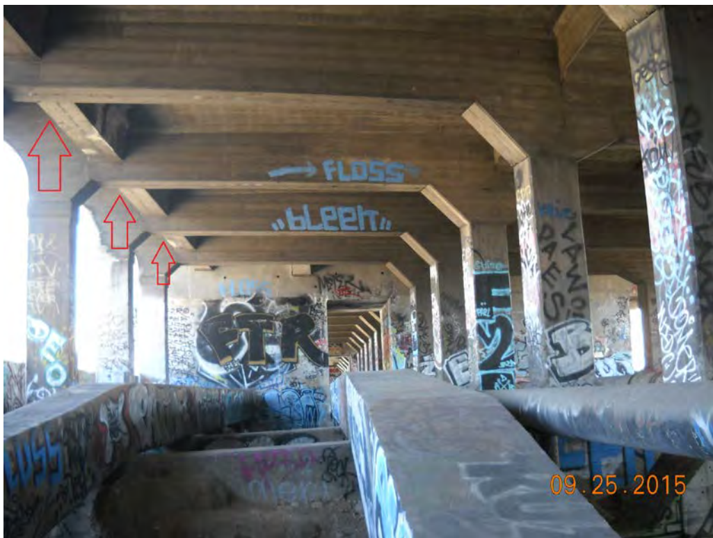
Photo 10: Approximate locations selected for placement of alternative bat habitat enclosures on the concrete girders (facing out towards the river channel) of the Seventh Street Viaduct; view facing east
