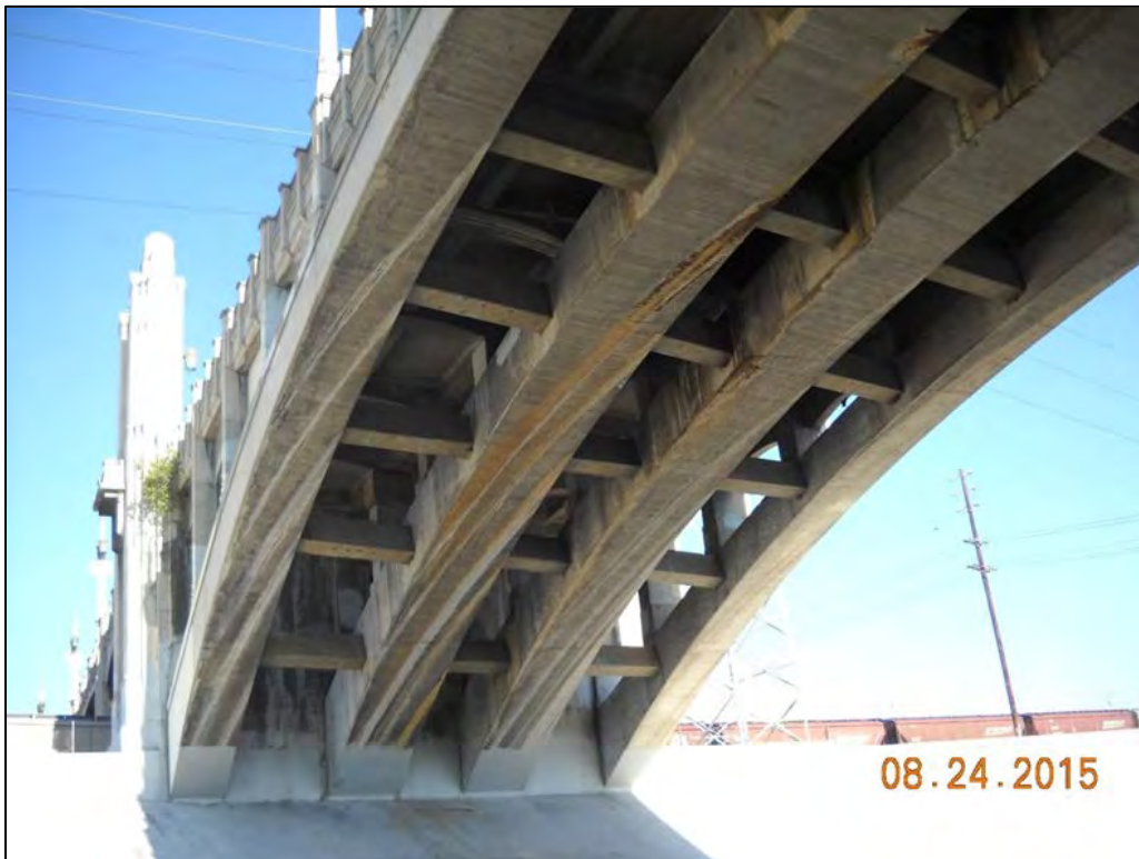
Photo 2: Underside of Fourth Street Viaduct showing concrete arches and girders; view facing east
