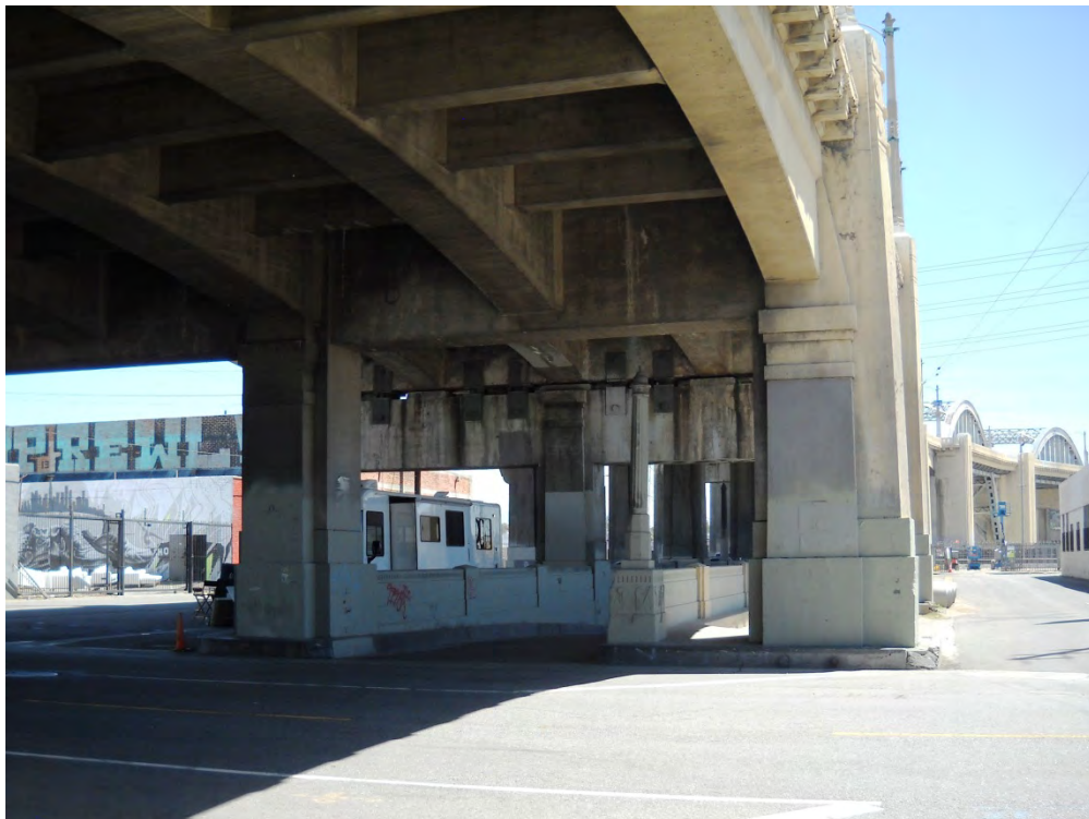
Photo 2: Solid concrete girders on viaduct with metal arches in the background; view facing east
