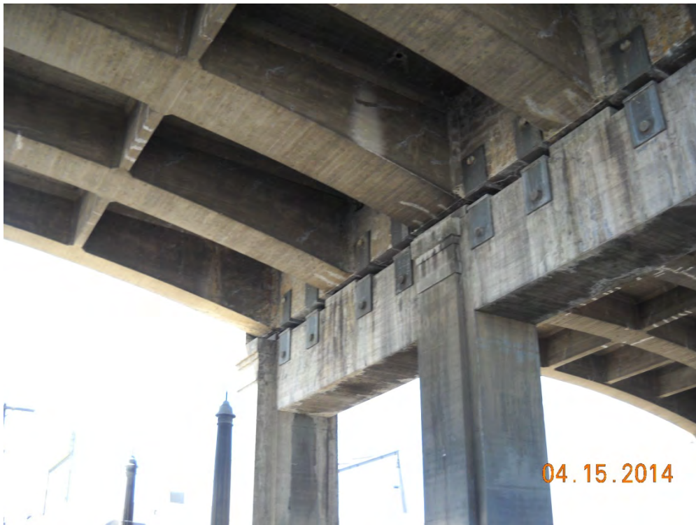
Photo 4: Pier support and metal bearings on viaduct, and an expansion joint providing suitable bat roosting habitat; view facing west
