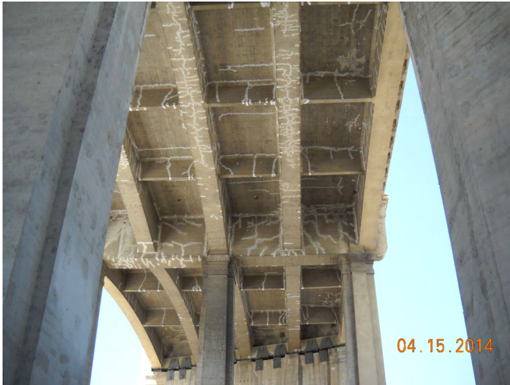
Photo 3: Sealed cracks on viaduct, cracked from alkali-silica reaction; view facing west
