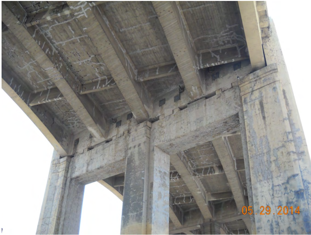
Photo 5: Pier support and bridge deck attachments on viaduct; and an expansion joint accessible to bats; view facing west
