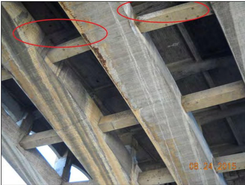
Photo 4: Underside of Fourth Street Viaduct showing western expansion joint; view facing west
