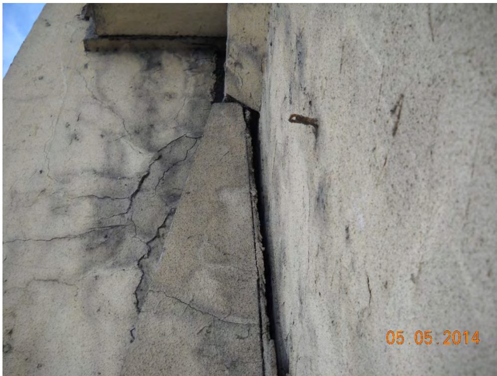
Photo 6: Crack on edge of viaduct near pier support wide enough (greater than 0.50 inch) to provide suitable bat roosting habitat; view facing west
