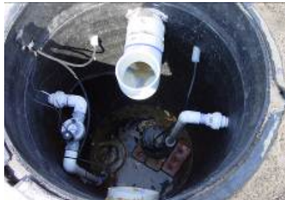
Figure - Reservoir access showing pump, float, & drain
