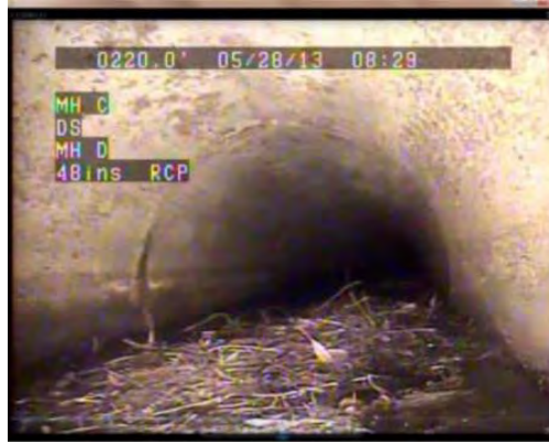
Figure 3. Clogged 48" RCP dated 2013
