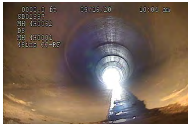
Figure 4. Unclogged 48" RCP dated 2020
