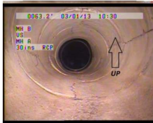
Figure 1.5B – Longitudinal cracking in 30” RCP. This 30” RPC is downstream of the 24” HDPE per the operator’s verbal comments and survey reports (see Appendix G).
