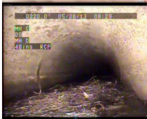
Figure 1.5A – 50% pipe clogging in the 48” RCP
