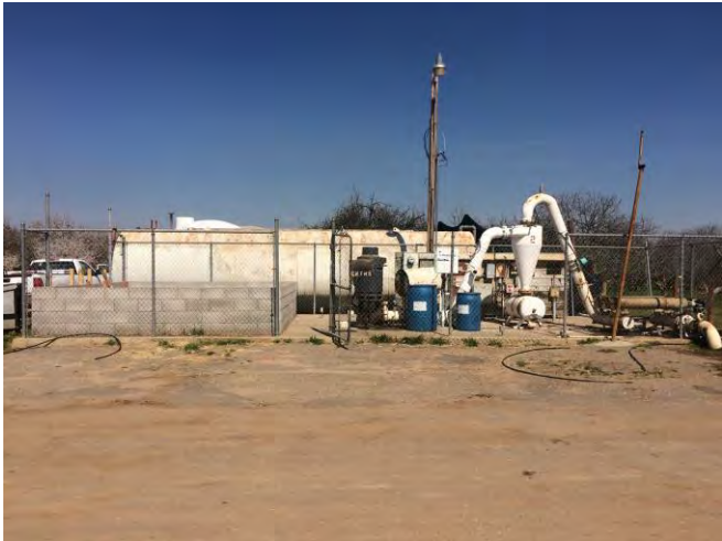
Well #2, View Facing North
