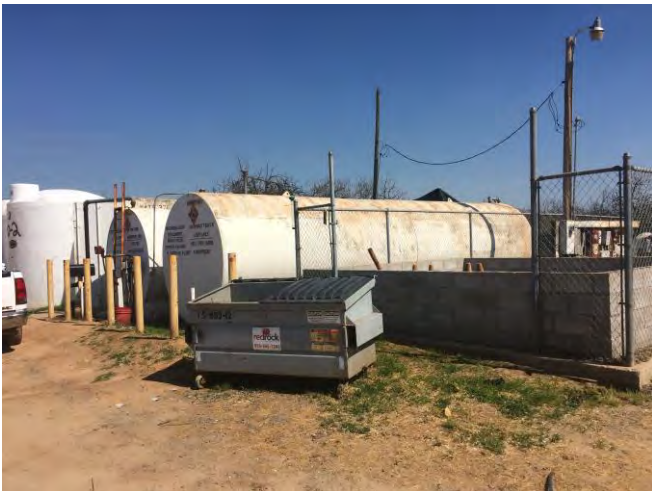
Diesel ASTs East of Shop Building View Facing Northeast
