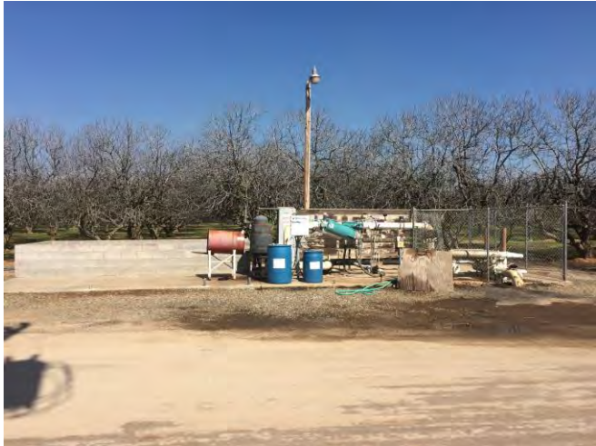
Well #4, View Facing North
