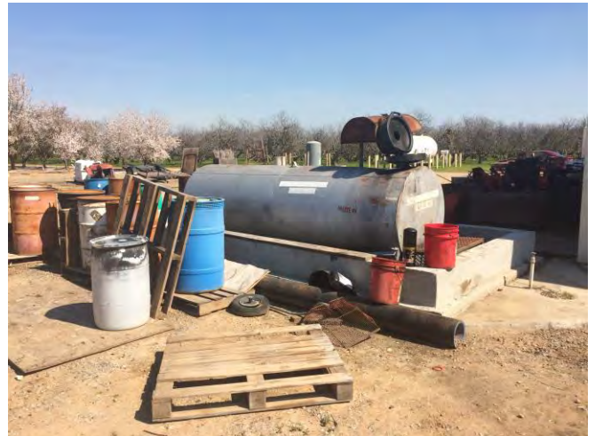
View of Waste Oil Tank, Containment & 55-Gallon Drums
