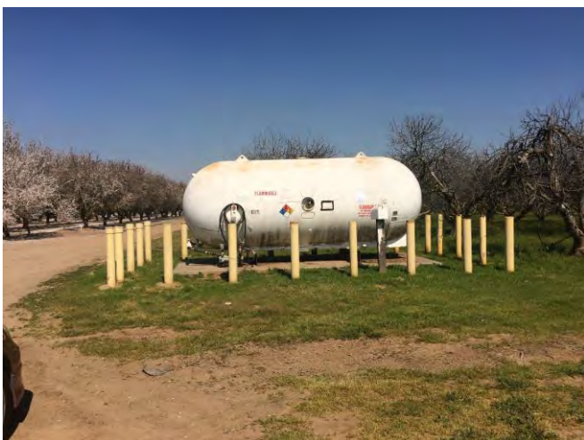
View of Propane AST View Facing North
