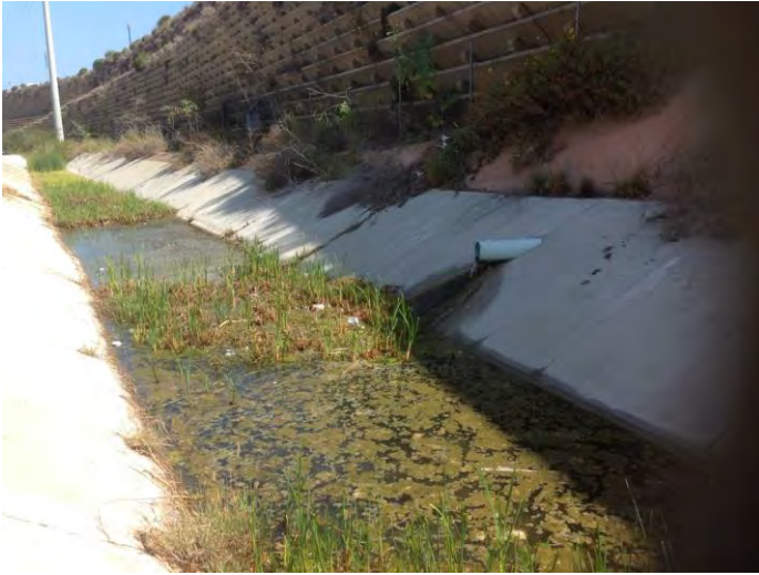
Storm drain channel that drains to Tripp Ct. Outfall. The channel receives continual groundwater seepage from retaining wall along I-5.
