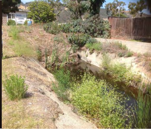
Storm drain channel that drains to Tripp Ct. Outfall. The blocked outfall creates standing water in the channel.
