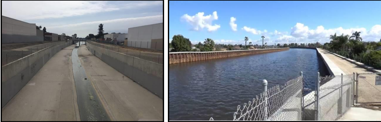
Figure 34: Examples of channel reaches with rectangular cross-sectional geometry to increase capacity and improve conveyance efficiency. On the left is a typical concrete lined rectangular channel. On the right is a soft bottom rectangular channel constructed using steel sheet pile walls.
