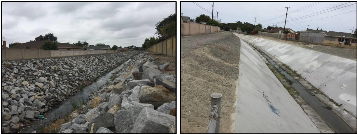
Figure 33: Typical existing trapezoidal channels. The picture on the left shows a typical existing riprap lined trapezoidal channel in the study area (before). On the right is a trapezoidal channel lined with concrete to improve conveyance efficiency (after).
