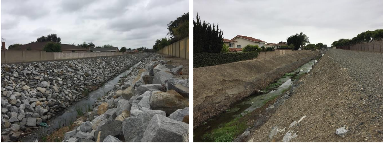
Figure 9: Riprap lined trapezoidal and earthen trapezoidal channels found within the Westminster watershed.
