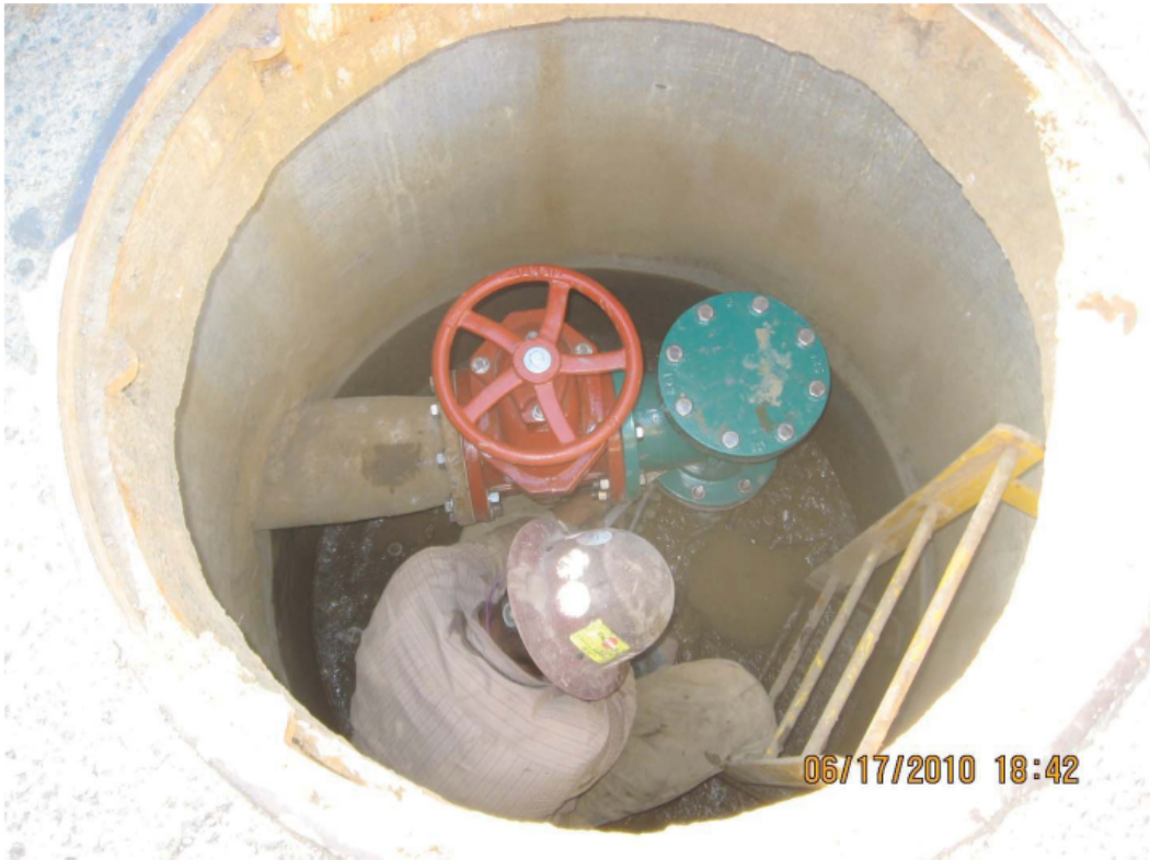
New blow-off valve installed during Phase 1 of the SCPL Improvement Project.
