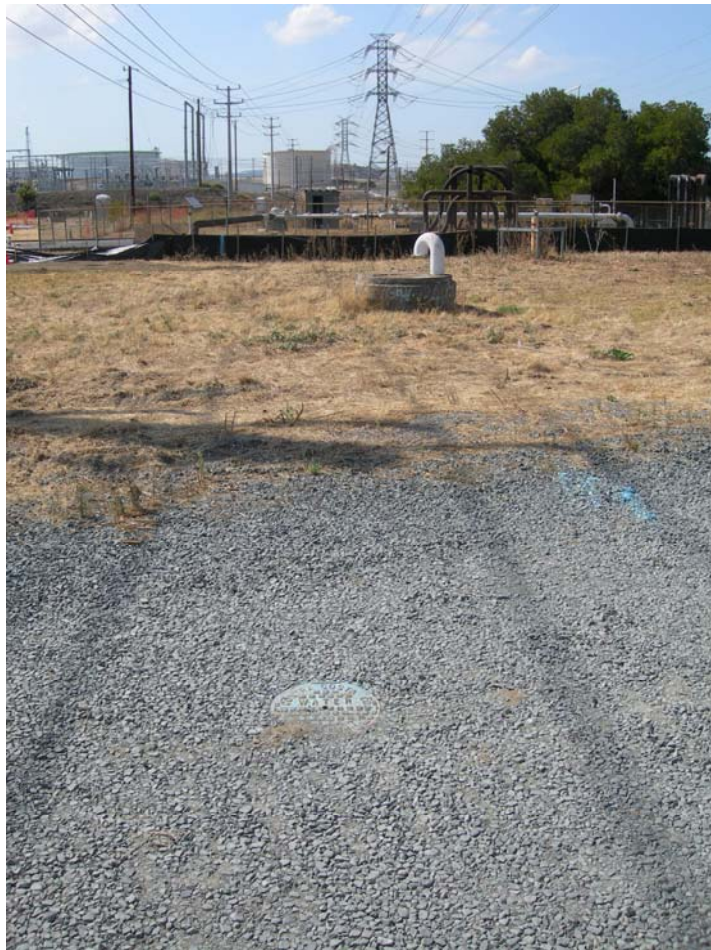
Example of a Butterfly can lid (in foreground) with Air Valve in background located at Site 6, within Tesoro's Waste Management Unit 4 (WMU4).
