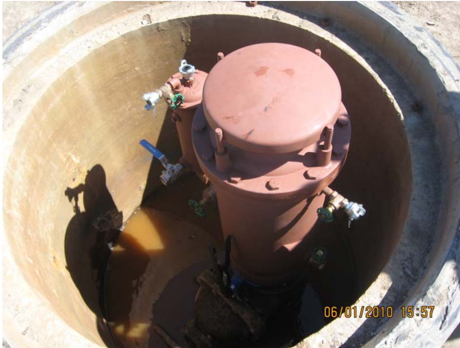
New interior Air Valve installed during Phase 1 of the CPL improvement Project on the Tesoro Refinery property.
