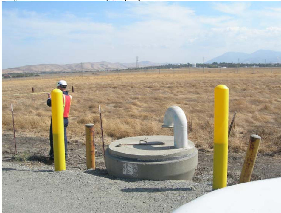
Typical Air Valve housing, located at the SCPL Site 8.
