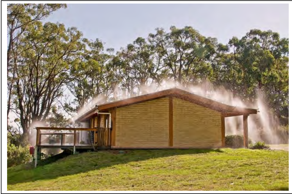
Figure 10. Exterior Sprinklers. As a wildfire approaches, exterior sprinklers wet the structure at risk, the surrounding environment, and increase humidity to prevent ignition. Photo: Platypus Fire Pty Ltd.
