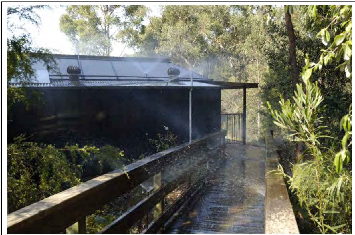
Figure 11. External sprinklers. As a wildfire approaches, external sprinklers wet the structure at risk, the surrounding environment, and increase the local humidity to prevent ignition. Photo: A conference center in New South Wales, Australia.
