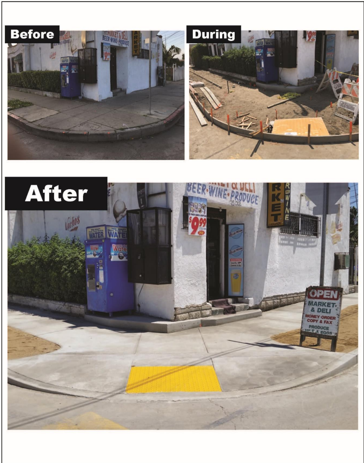
Figures 2-4a. Sidewalk Repair – Before and After
